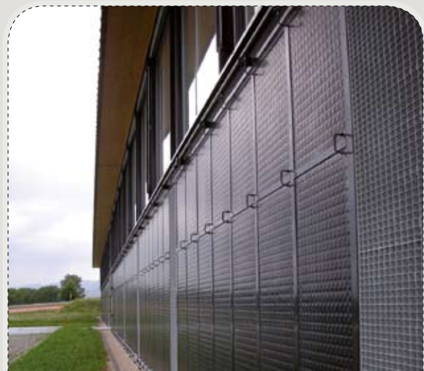
FIGURE 9: Details of the interconnection of the stainless steel collectors and connection to the upper tube for the heat transfer fluid
