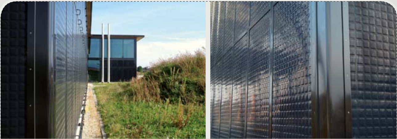
FIGURE 8: Partial view of a non-active facade. The stainless steel elements are visible below the windows of the upper floor (left).
