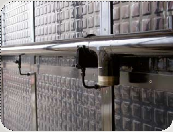
FIGURE 12: Close-up of the connection of the collectors to the upper tube for heat transfer fluid
